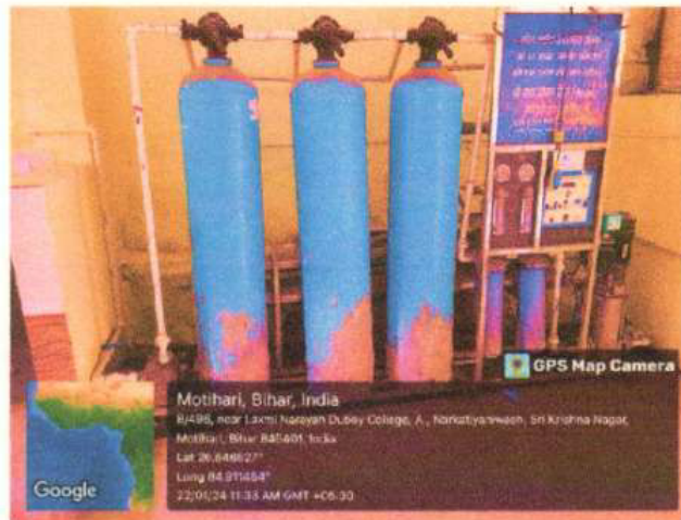
RO PLANT at L.N.D. College
