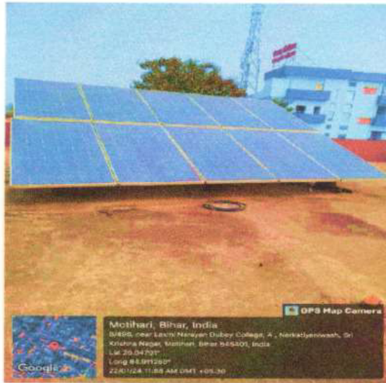
Solar Roof Top Panel installed at L.N.D. College
